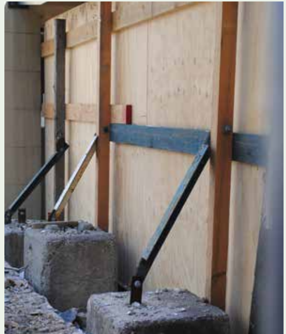
Figure 3.37: Typical concrete block counterweight with lateral bracings.
